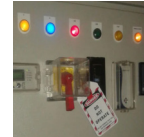
Electrical Panel Lockout
